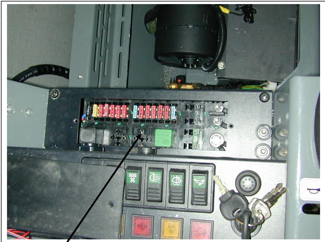
Terminal with ignition live power
